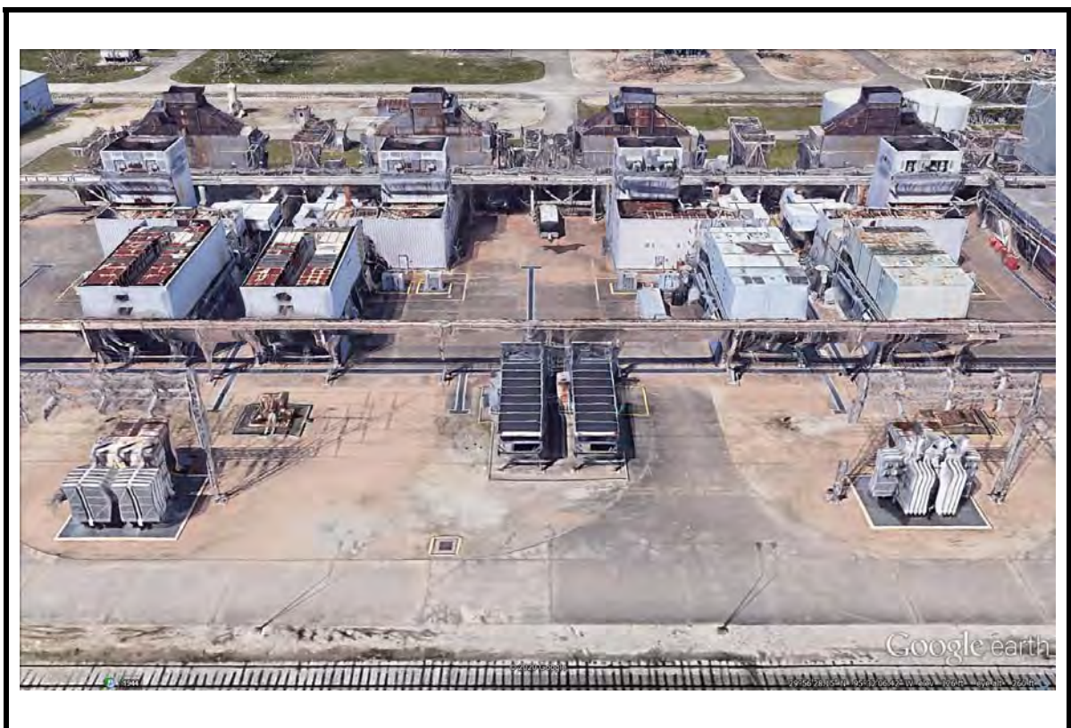
Photo 6: Gas Turbines 41, 42, 43, and 44, facing north.
