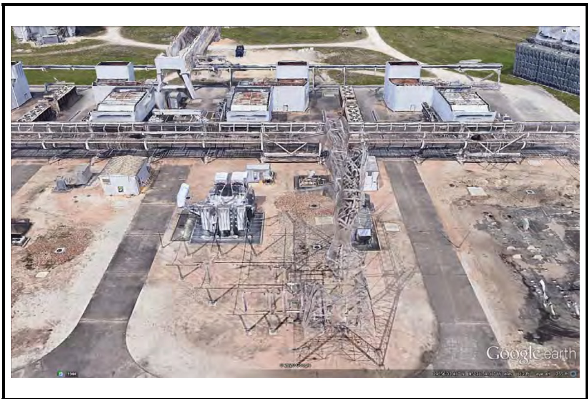
Photo 7: Gas Turbines 51, 52, and 53, facing north.
