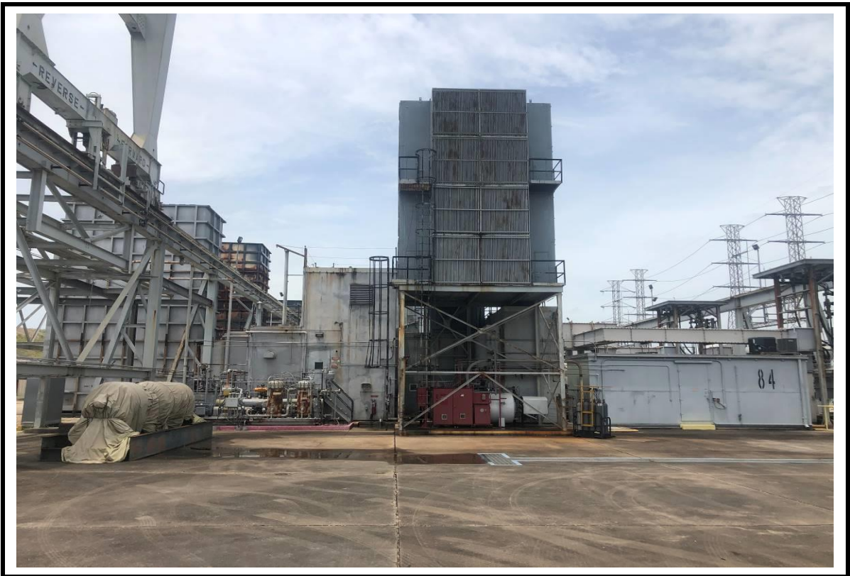
Photo 8: Gas Turbine 84, facing north.
