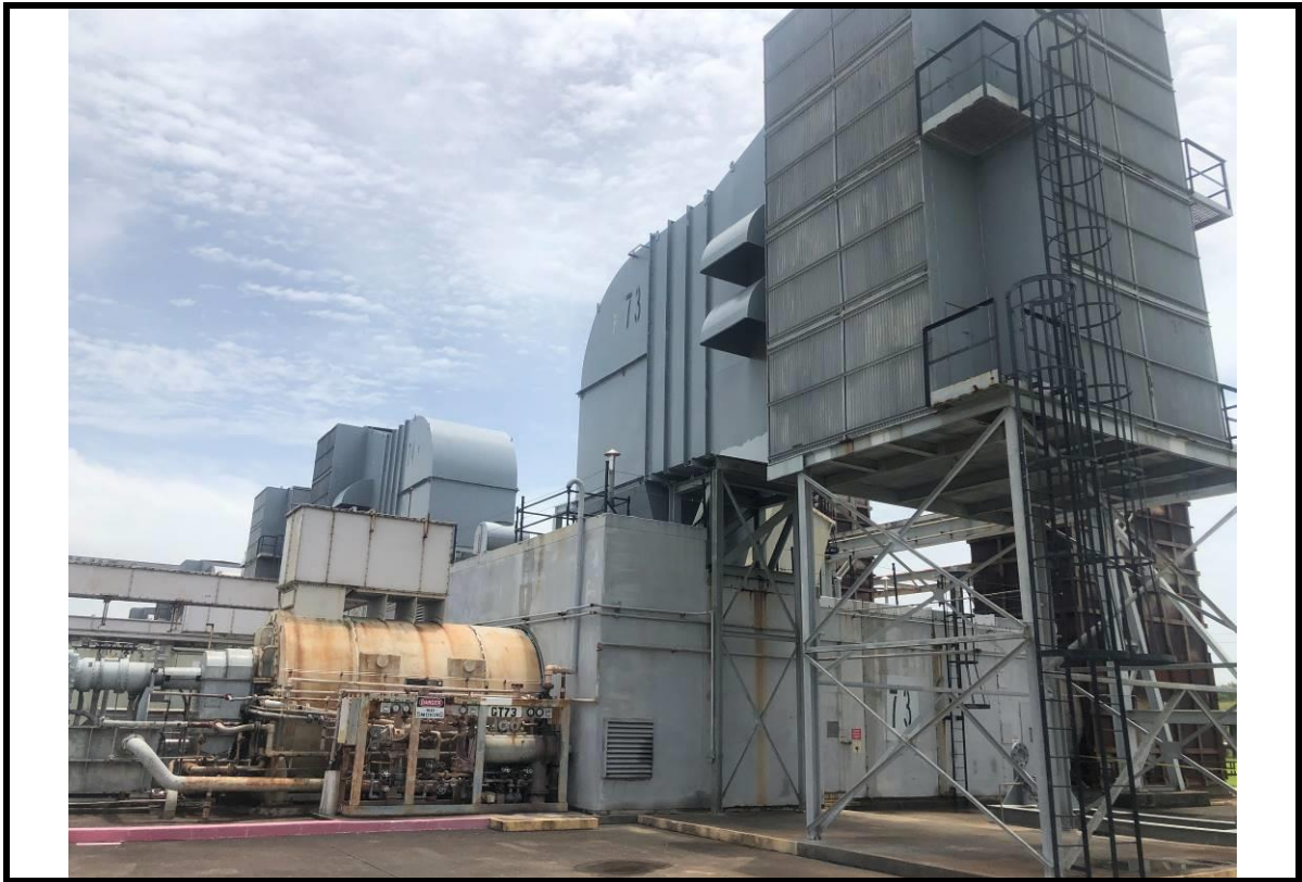
Photo 5: Gas Turbine 73, facing northeast.
