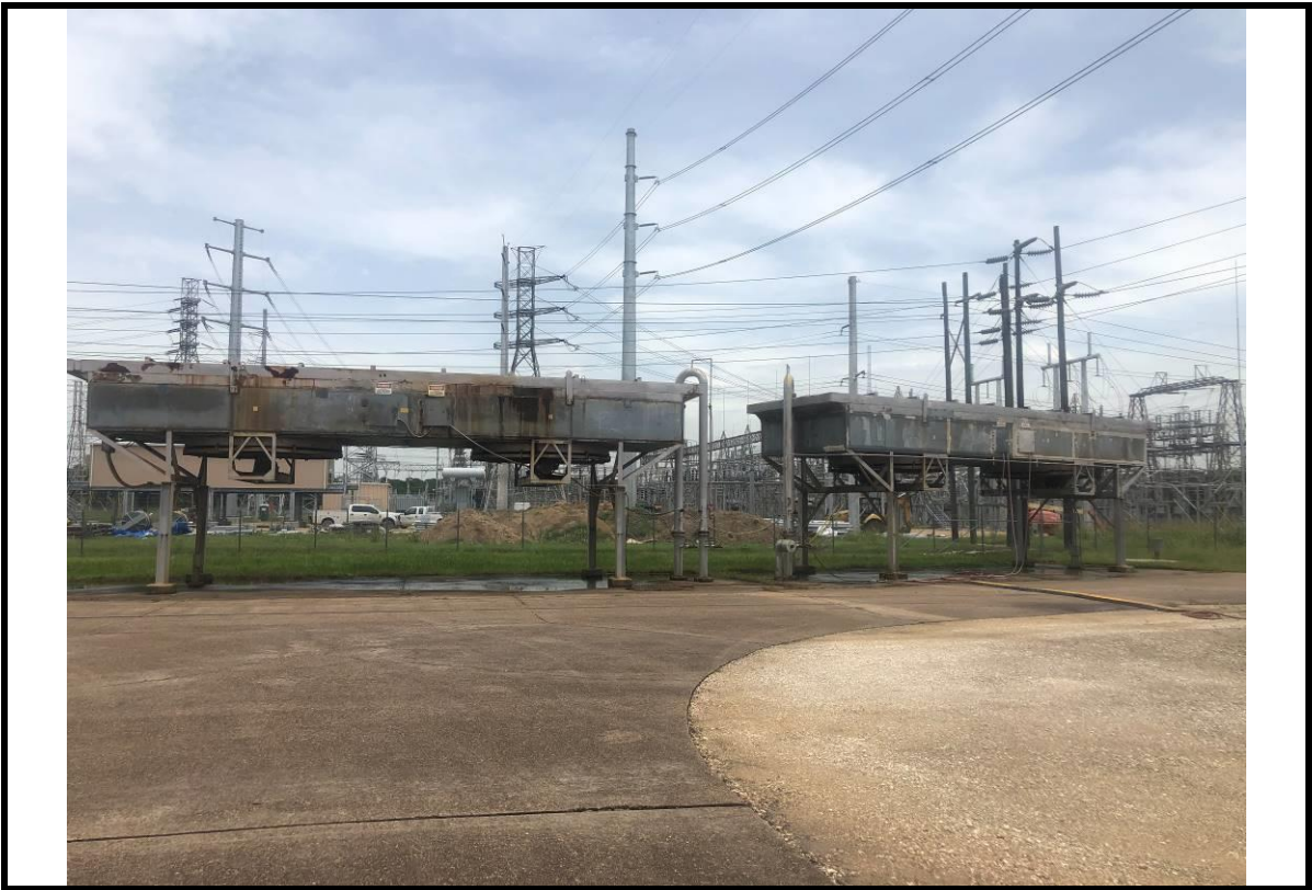
Photo 7: Gas Turbines 83-84 Cooling Skid, facing east.
