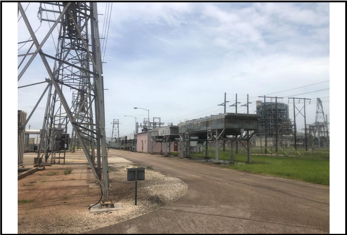
Photo 9: Gas Turbines 81-84 Cooling Skid, facing northeast.
